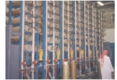
Hollow fiber membranes being used to desalt brackish water near Riyadh, Saudi Arabia
