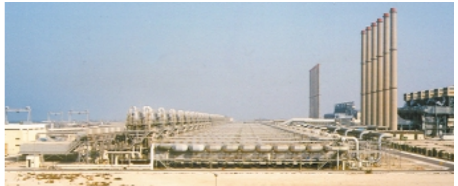
Dual purpose (power-water) facility in Saudi Arabia
