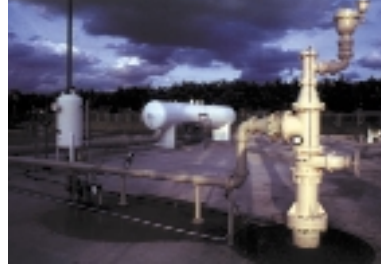
A deep disposal well for RO concentrate in Florida. The surge tank for the system is in the background
