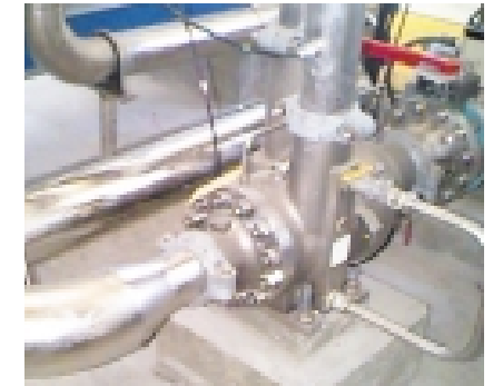
Interstage energy recovery unit integrated with the pump
