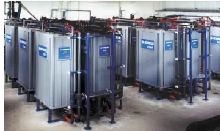
A 4,000 m 3 /d (1mgd) EDR unit, Port Hueneme, USA Photo — Ionics
